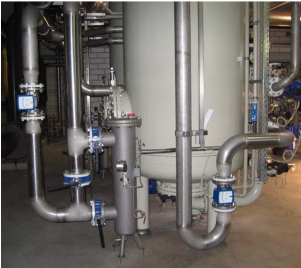
Condensate polishing line with resin trap
