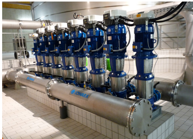
Pressure booster system with frequency converters
