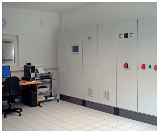
Control center in a waterworks
