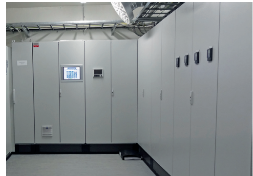
Central control cabinet in a waterworks
