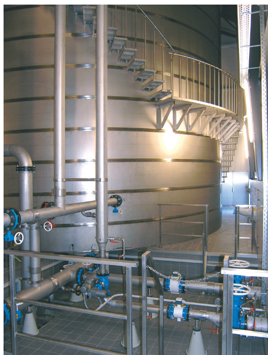
Stainless-steel tank system with installation
