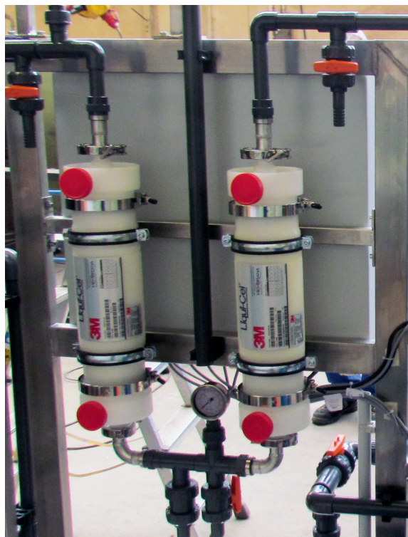
Two-line system with membrane degassing units
