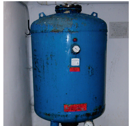
Fig. 2: Corrosion and rust
