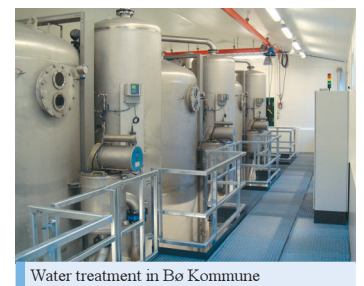
Water treatment in Bø Kommune
