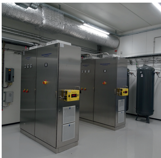
Figure 4: Ozone production systems in cabinet design
