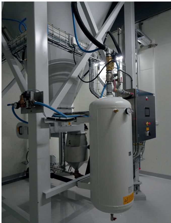
Figure 7: Lime silo with controls and water jet pump
