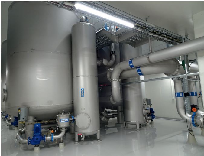
Figure 5: Filter vessel with ozone mixing and reaction system
